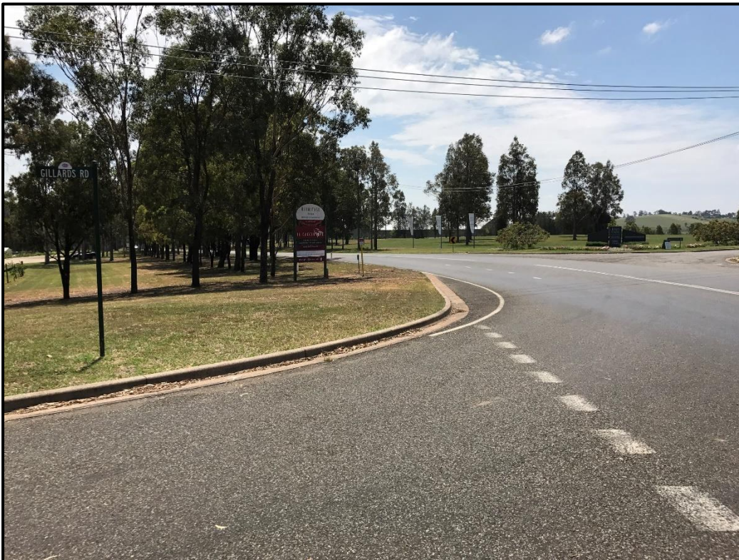
Photo 6 – Visibility looking left (north) along McDonalds Road from the intersection with Gillards Road. Shows existing vegetation adjacent to the road which restricts the sight lines for drivers turning onto McDonalds Road.
